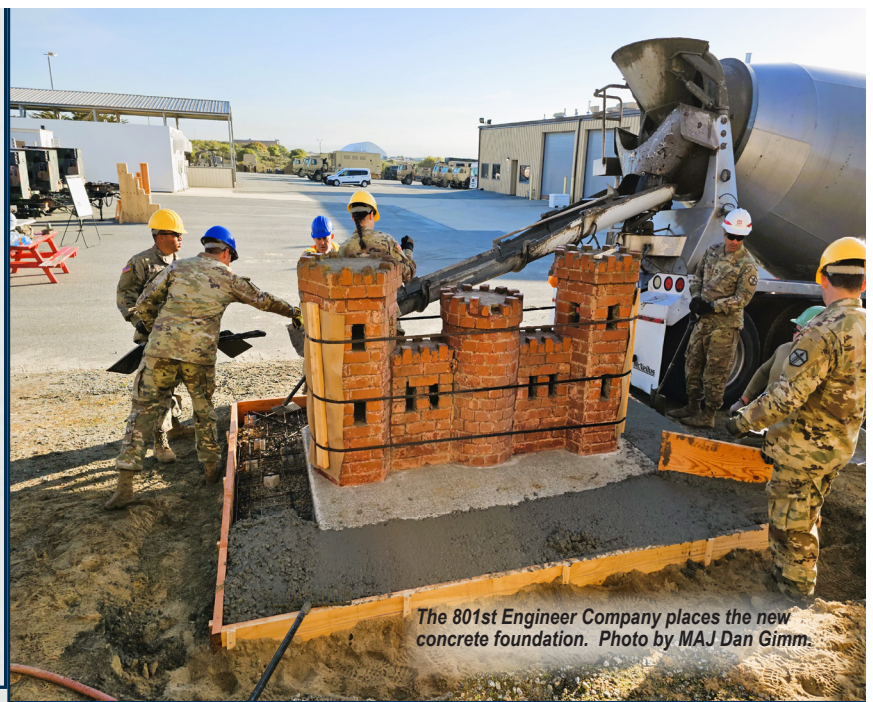
MAJ Gimm finishes the brick and mortar repairs. Photo by Derek LeBeouf.
