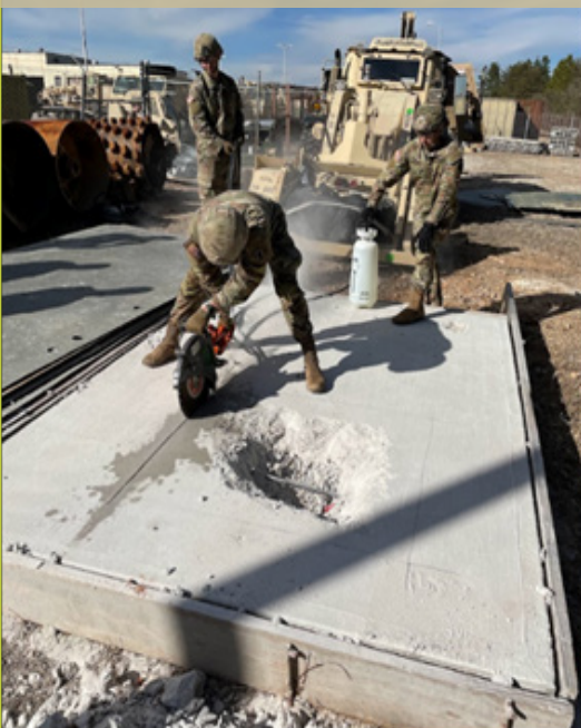
618th Engineer Support Company (Airborne) Paratroopers train on concrete cutting using hydraulic power from the HMEE. Photo by 1LT Ross Caywood.
