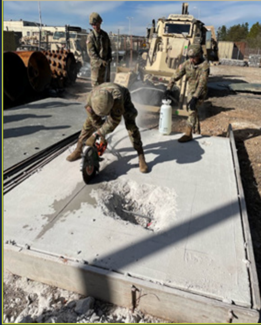
618th Engineer Support Company (Airborne) Paratroopers train on concrete cutting using hydraulic power from the HMEE. Photo by 1LT Ross Caywood.
